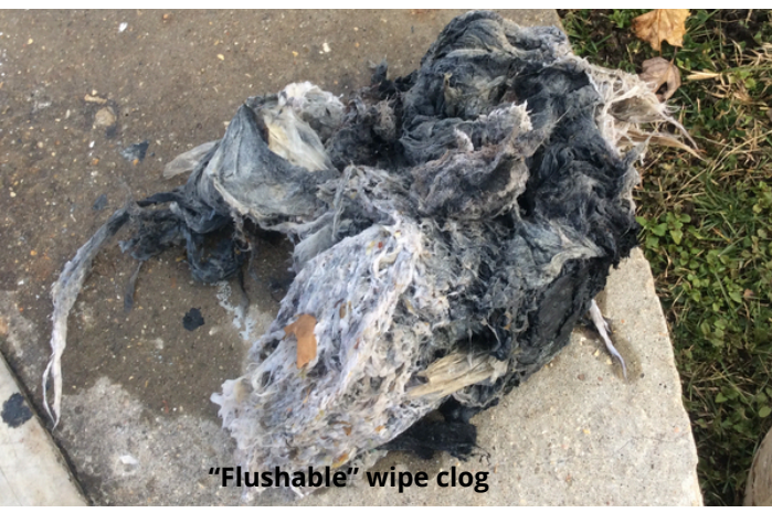
"Flushable" wipes stuck in a lift station pump
