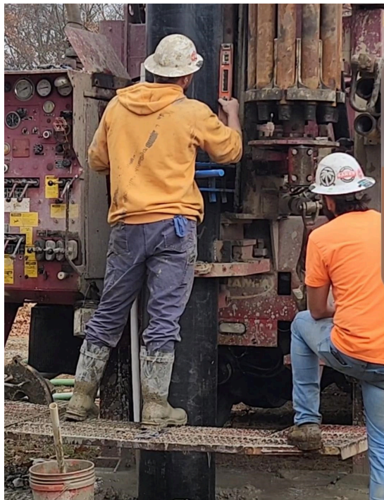
The crew checking the well casing (a pipe installed vertically to stabilize the soils around the hole down to the ground water) that will be placed in the bore hole from ground surface down to and into the bedrock below.
