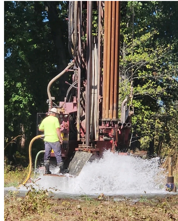
Dyer Well Drilling crew in the process of drilling in the deep aquifer. During this process, the rock and soils that are being drilled out of the various layers of the earth are brought to the surface with the combined power of water and air forced through the drilling bit.
